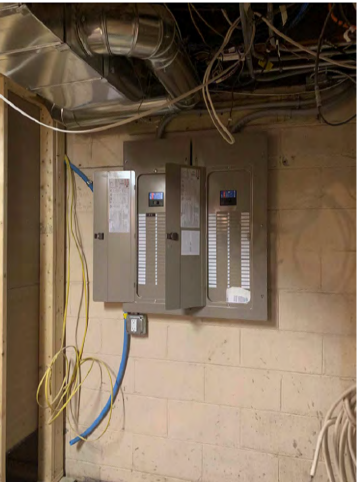
Main service panel in basement.
