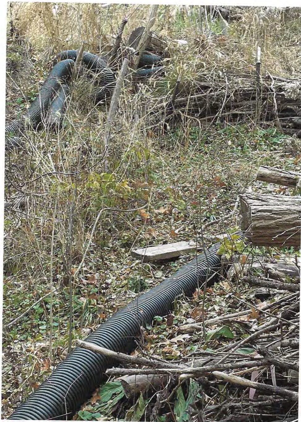
LOCATION 1 - TANGLED DRAINS CAUSED BY BLUFF SLIDE ABOVE
