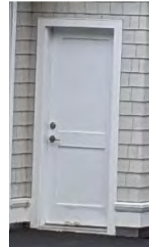
Pool Equipment Man Door
