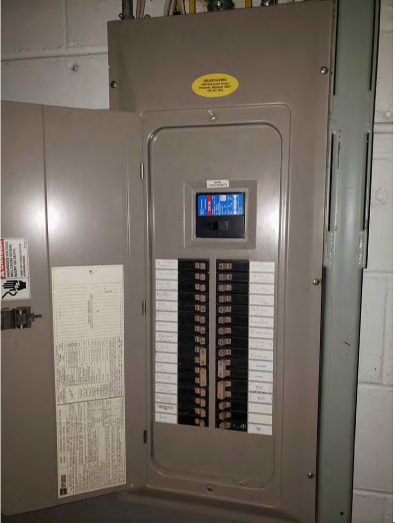
Main service panel in basement.
