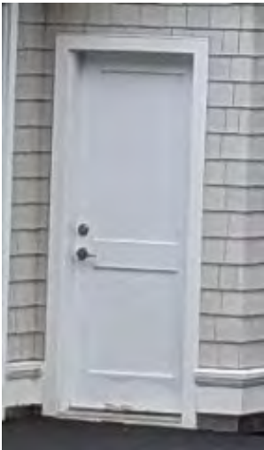
Pool Equipment Man Door
