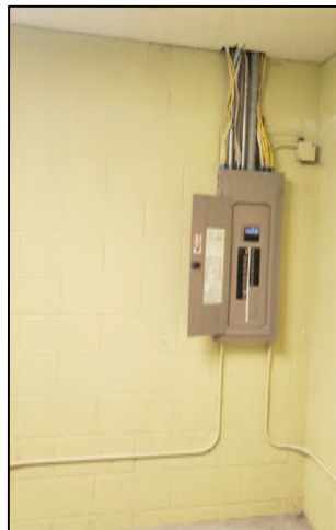
Main Panel Located in basement.
