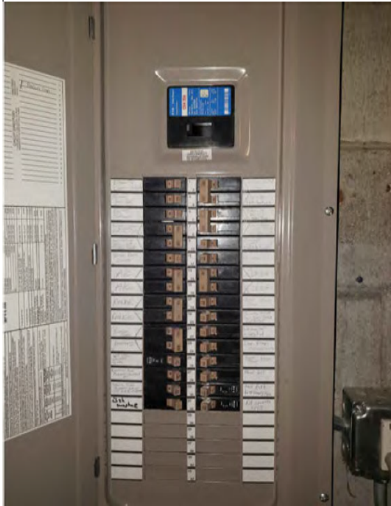
Main Panel Located in basement.
