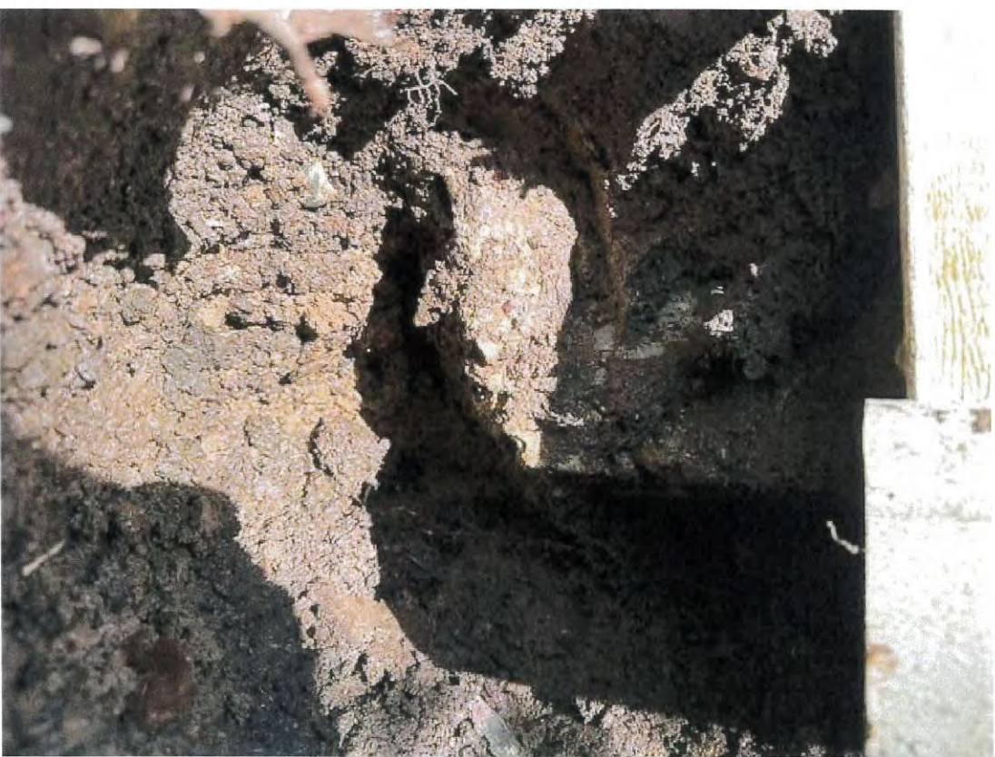
Corner of Garage Slab - Approx. 10"
