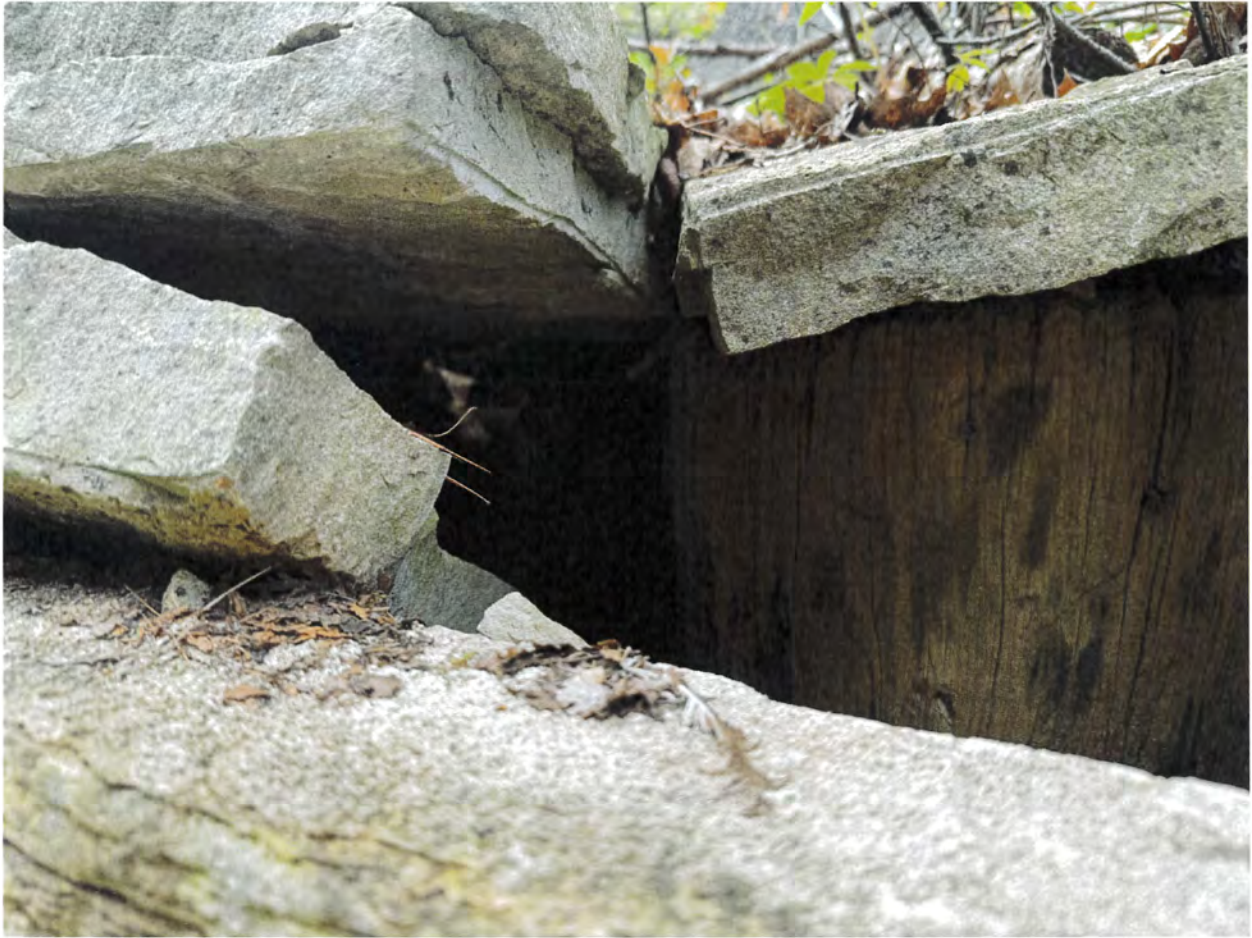
Image 4 – Retaining Wall 7900 block Beach Drive – April 2026
